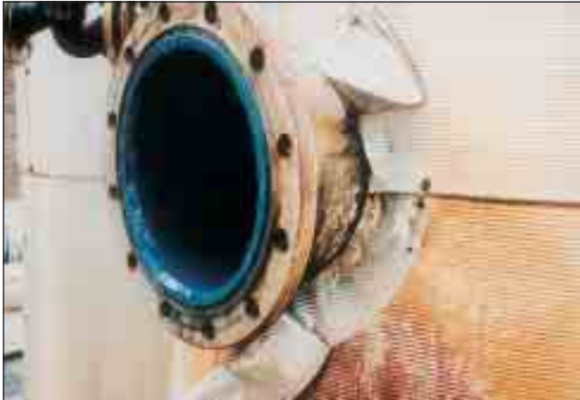
Picture 1 Entrance of CO 2 installation
